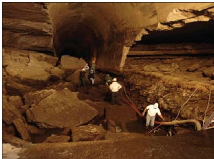
▲ Years of excess water events damaged the invert, as we saw when the tunnel was de-watered.
