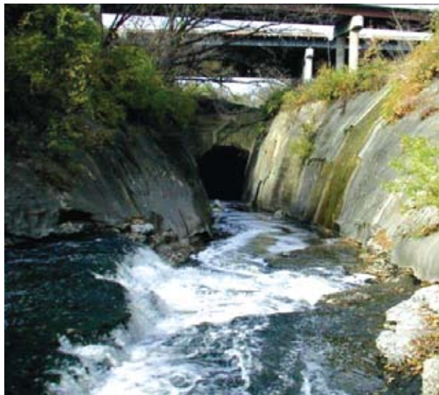
▲ This photo of the creek invert before construction shows the enormous amount of water the tunnel receives, as well as the difficulty crews faced getting equipment down the sides of the creek.
